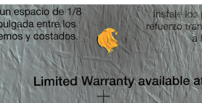
05 OVERDRIVEN FASTENER WITH DENSDEFY LIQUID FLASHING
