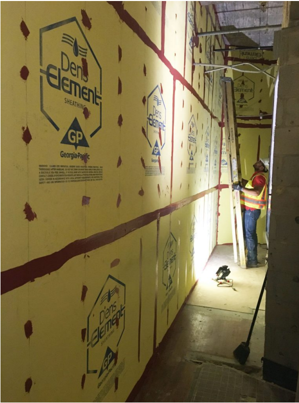
Image Pictured: Temporary Wall Holds Up to Hurricane Harvey: University of Texas Medical Branch in Galveston, Texas.
